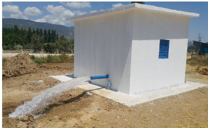
Drinking water well pump station
