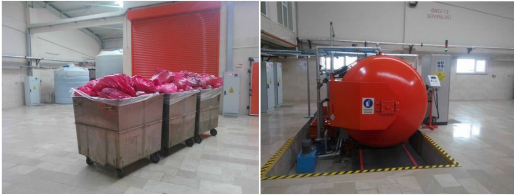
Waste transfer to the municipal sterilization facility
