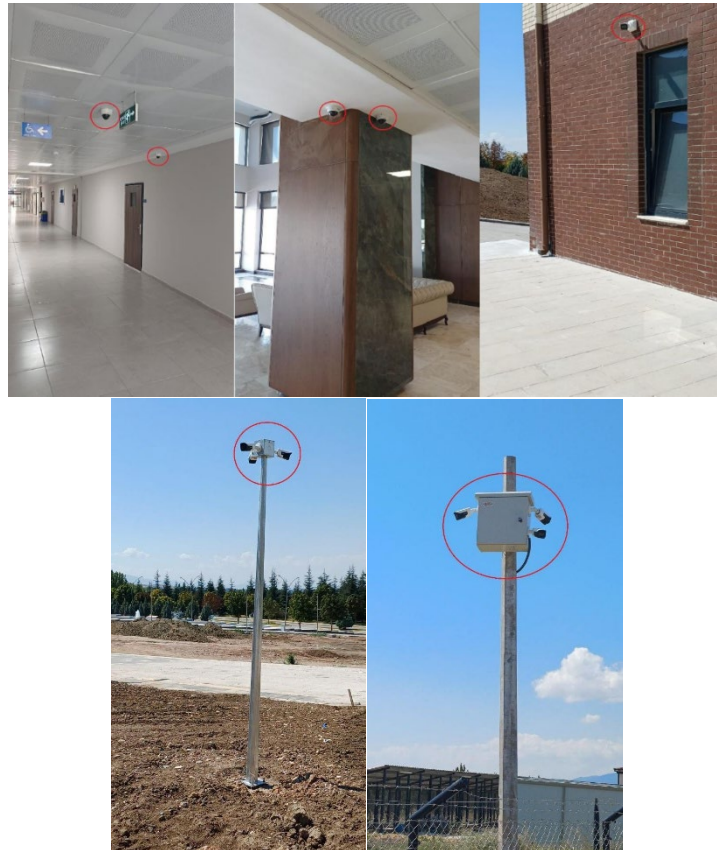
CCTV systems inside and outside buildings
