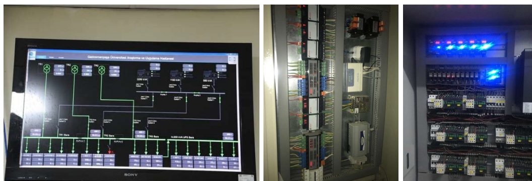
Energy monitoring and control system, PLC panel and power panel
