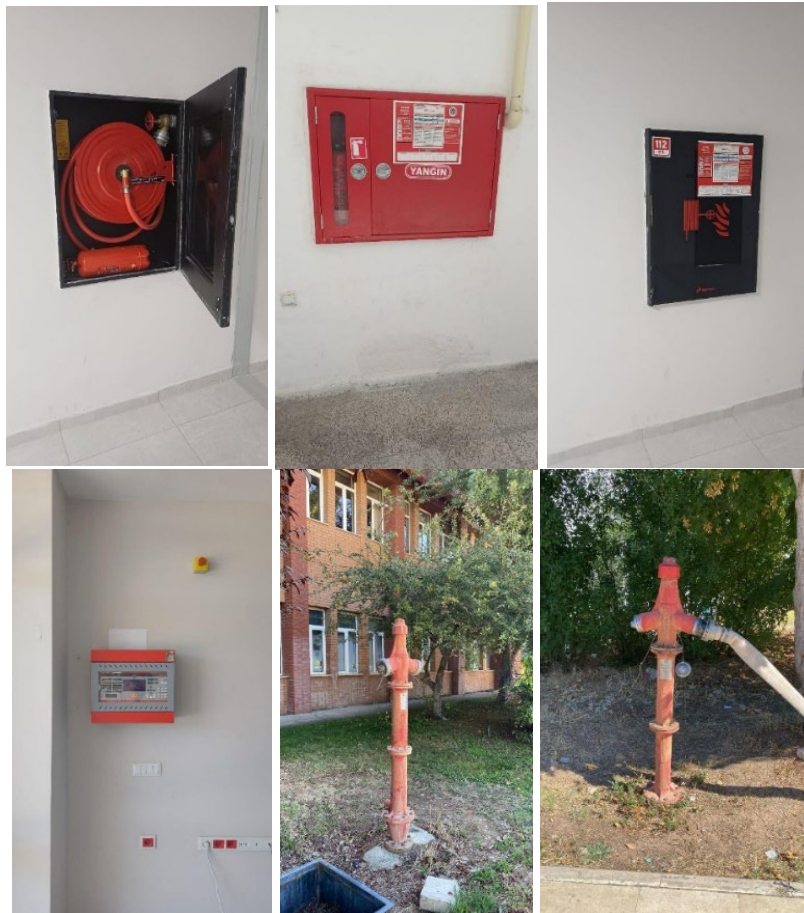
Fire hydrants inside and outside buildings
