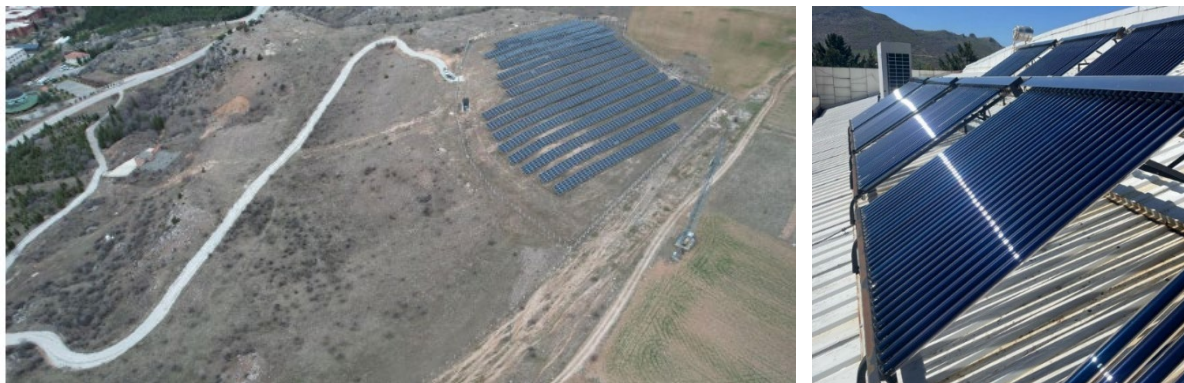
Solar Power Plant (left) and solar thermal panels for hot water generation (right)
