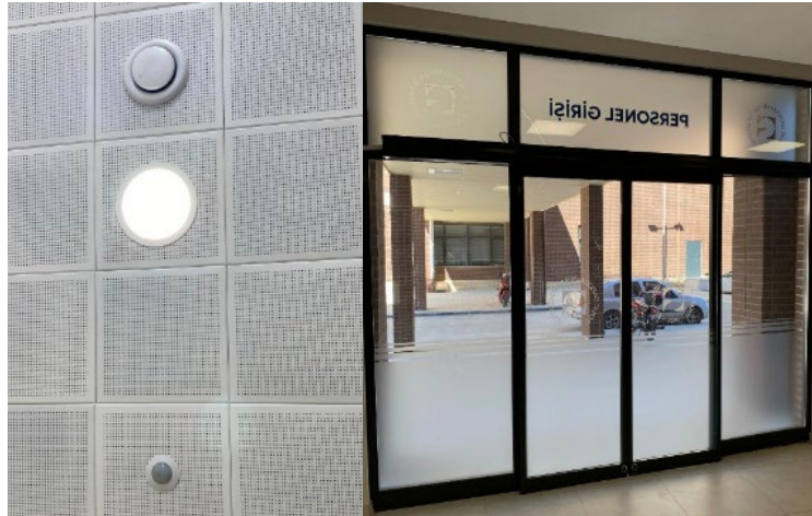
Photocell lighting sensors and automatic photocell sliding doors
