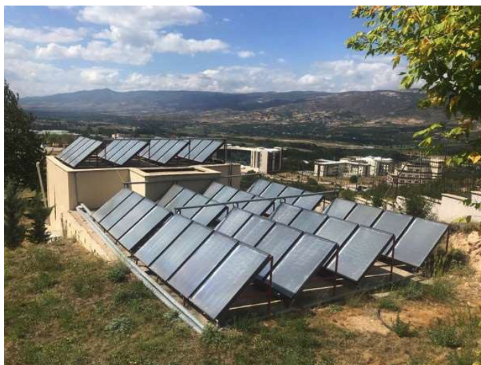
Solar thermal panels
