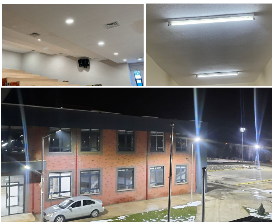
Energy-efficient LED luminaires
